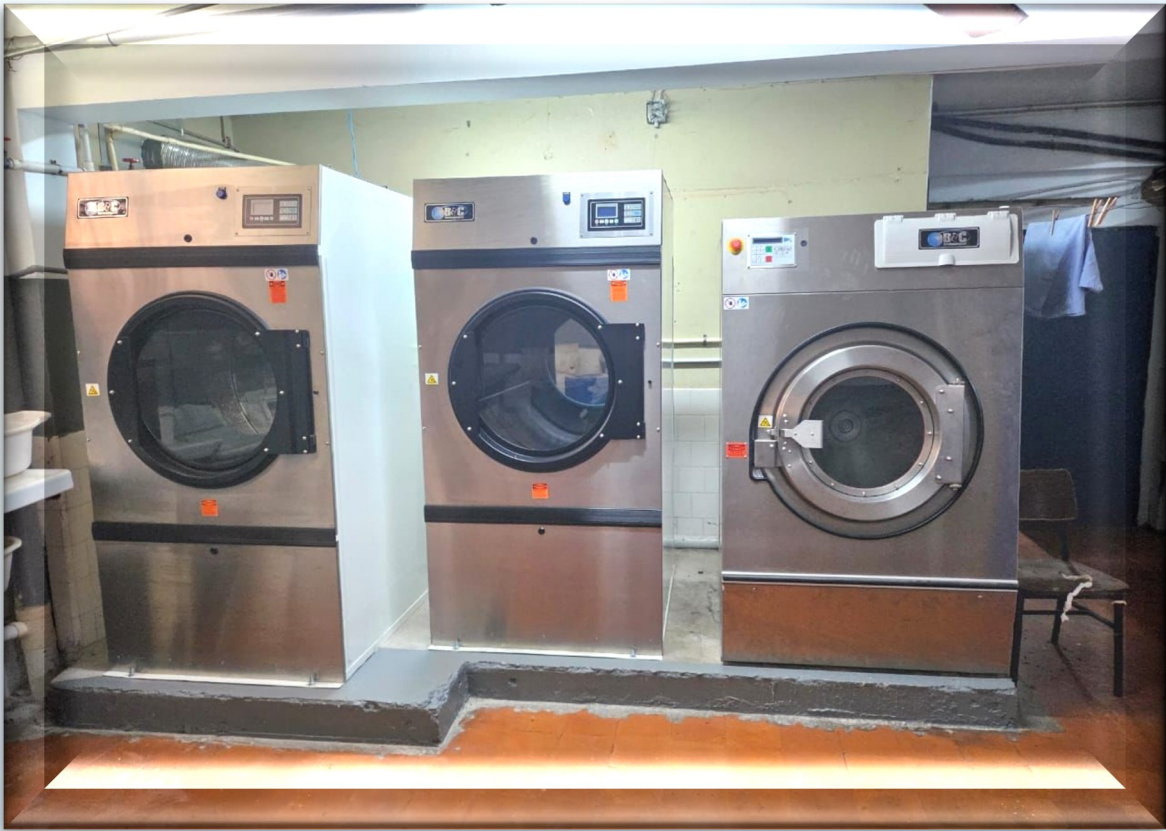
Photo of two dryers and one washer installed at the Victoria Jubilee Hospital
